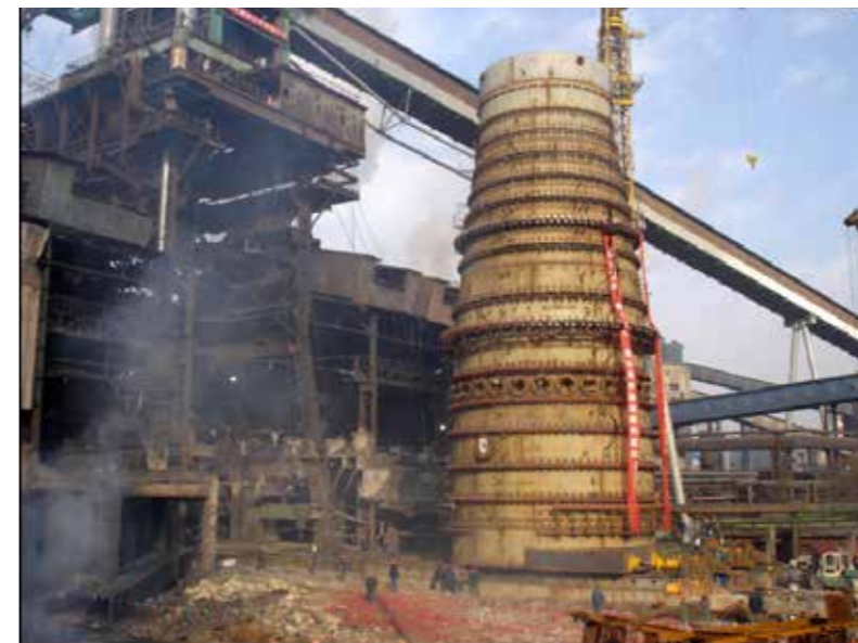
宣钢3号高炉(2000m 3 )整体推移前，推移重量4900t，推移距离37.78m
